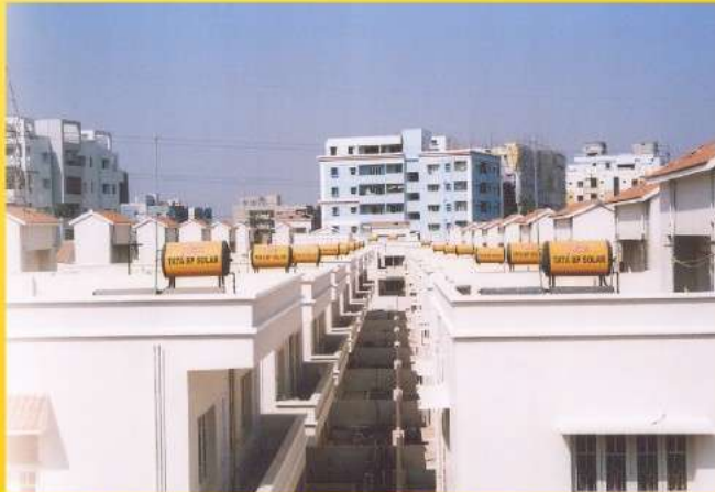
Zing Solar Water Heaters installed at Vasantha Estates, Hyderabad
